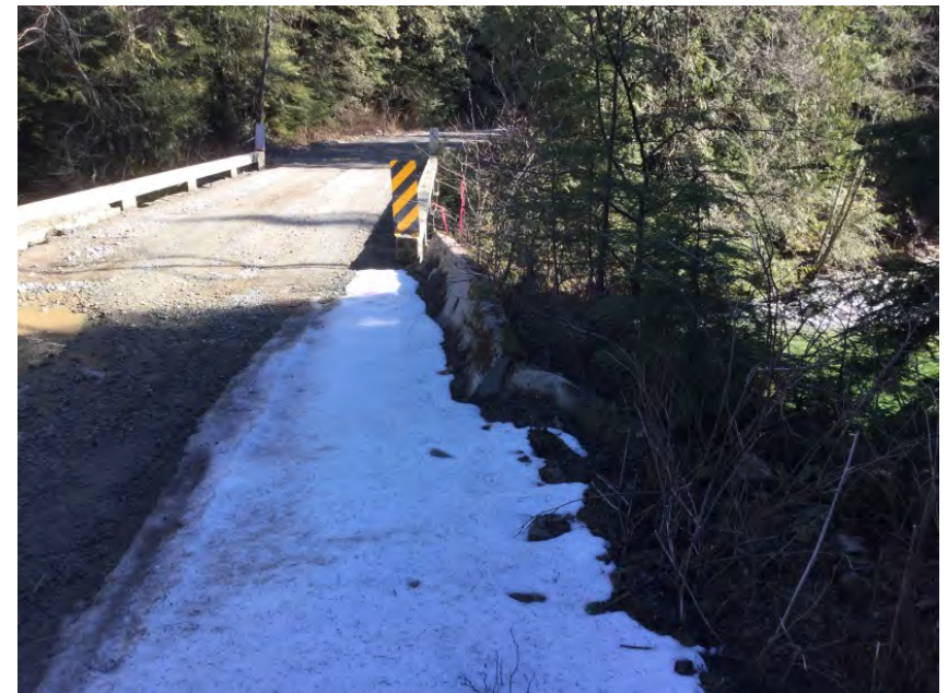
Downstream right approach no posts
