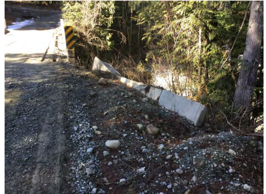
Upstream left approach no posts off road
