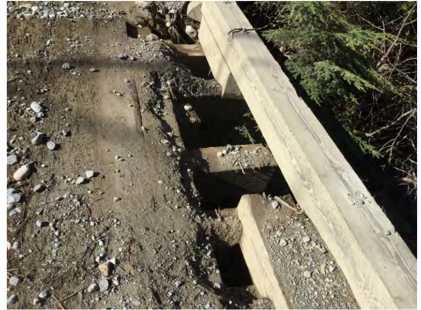
Tie alignment at right bank not consistent, upstream shown
