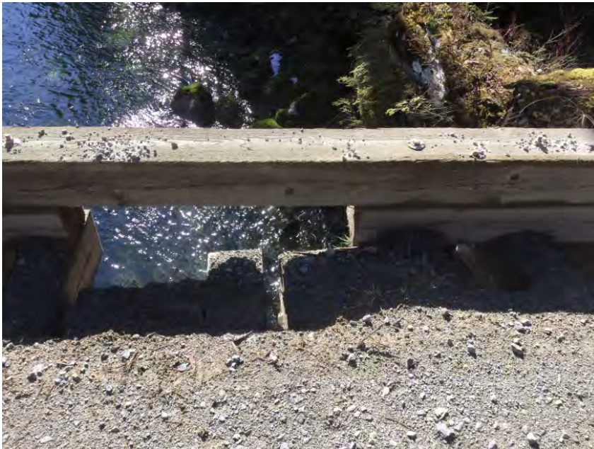
Tie alignment at right bank not consistent, downstream shown
