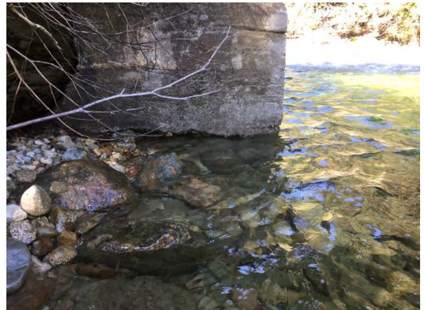
Scour under downstream right bank CIP does not appear any worse
